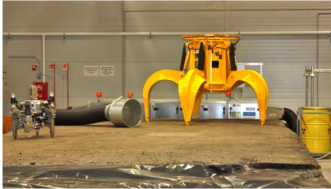
Covered Maišiagala radioactive waste cellar and part of the radioactive waste retrieval equipment
