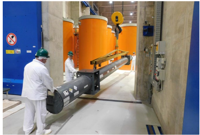
Placing unused nuclear fuel in SFSF-2
